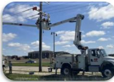
SUN PRAIRIE UTILITIES
