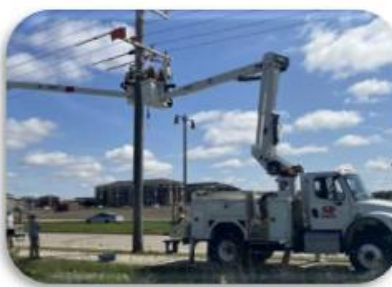
SUN PRAIRIE UTILITIES
